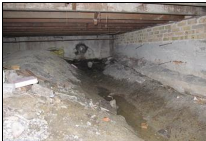
Water pooling right crawlspace. Copper water line running along this area
